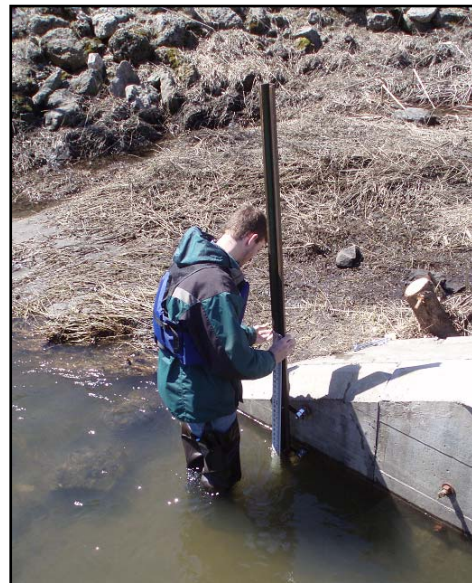
Installing the staff gage on the culvert at Blooming Prairie Tributary where it crosses Mower County Road 2.
