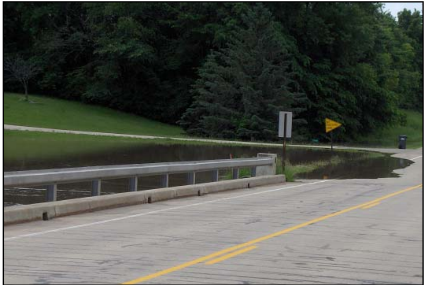
Water rising during the June 2008 flood on Rose Creek at Mower County 29
